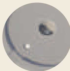
OVERFLOW HOLE AND RESERVOIR DRAIN HOLE
